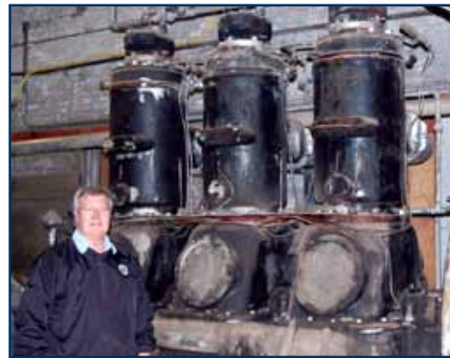
Louisburg Utility Director Ray Patterson in front of antique diesel generators housed at the town's old utility department.
