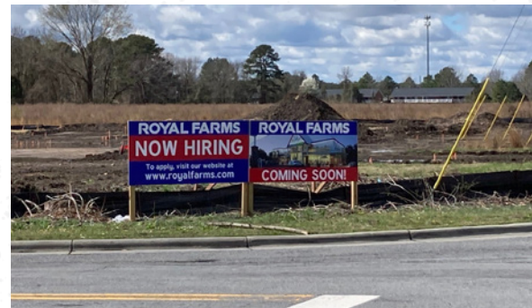
Development on this Royal Farms site in Greenville, North Carolina, is underway. Experts recommend that communities ensure their permitting processes are clear and consistent.
