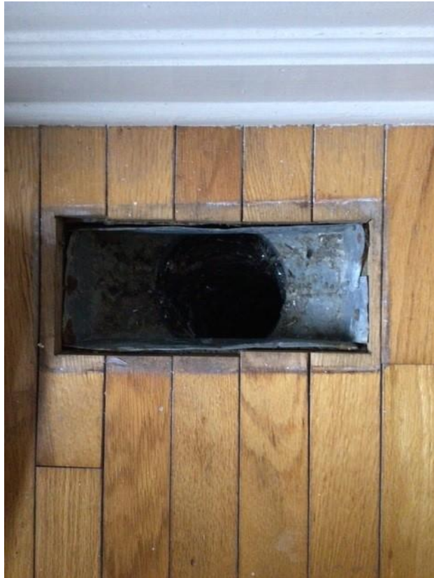
Disconnected supply duct
