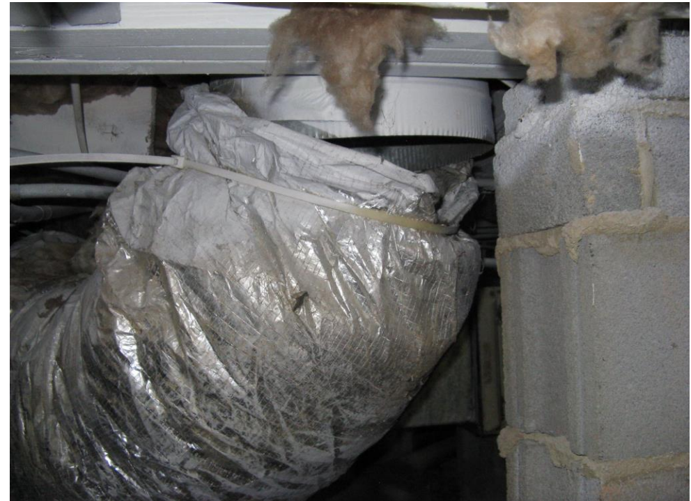
Unsealed collar connection
